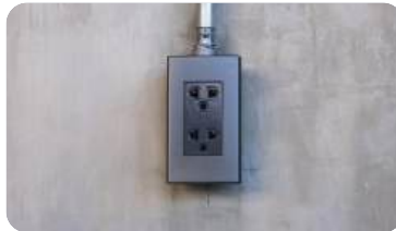
Plenty of In-Unit Outlets
